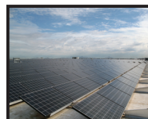
Gatorade Distribution Facility - Tolleson, AZ 500kW System Performing at 108%
